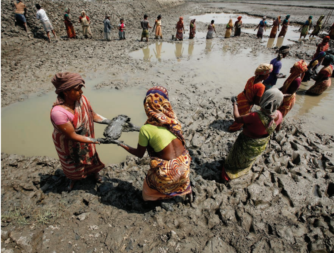
Women work to rebuild an embankment in one of the regions hit by Cyclone Aila in Dacope, Khulna, Bangladesh.
